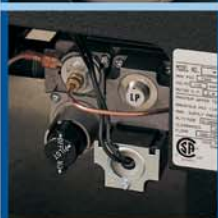
LP-gas shut-off valve
